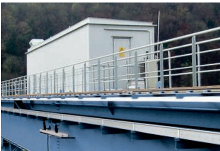
↑ The entire control system is installed in the electrocontainer to make maintenance easy
