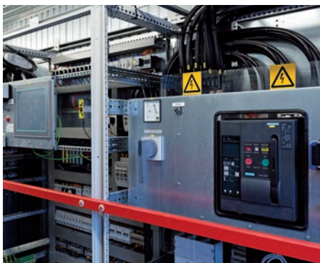
↑ Switch racks in the air conditioned electrocontainer
