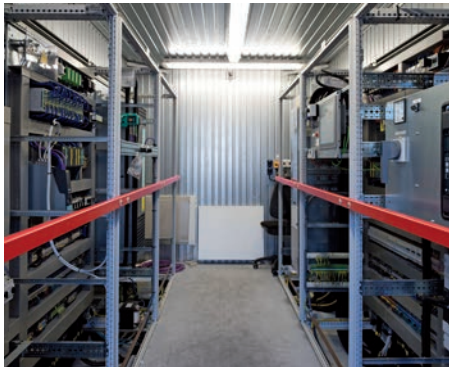
↑ Inside the electrocontainer
